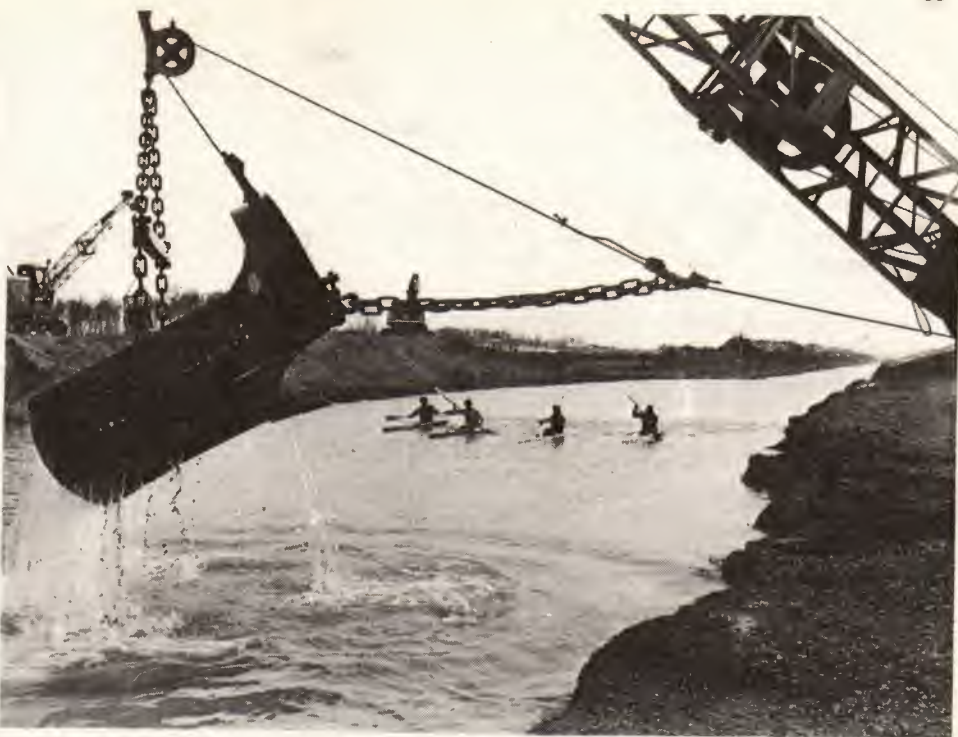
Canoeists try out the water during construction of the 2230m. Olympic regatta course 7½ km north of the Olympic Village at Munich. The course is now largely completed and the associated buildings, including a training hall, sauna bath, changing rooms and restaurant as well as boat houses, are expected to be completed early in 1972. Photo: Olympia Press.
