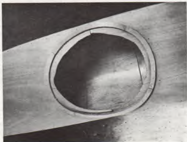
Three thicknesses of coaming ply fitted. Two more are to be fitted with an overlap for the spray cover.
