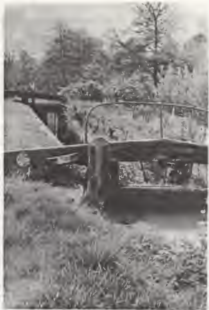
A "good" lock before repair.
