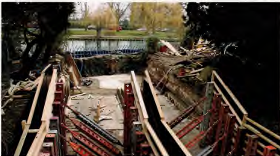
Above: The twin screw hydro under construction in the centre of Bedford.
