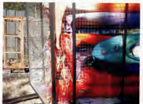
Above: The fire damage after the arson attack.
